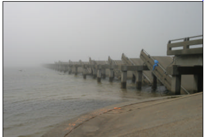
Damage from Hurricane Katrina
